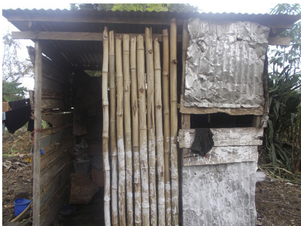
Fig. 8. Example of a plank house considered unsuitable for use with LPG (P3, F, age 45, Rural, Income 1).
