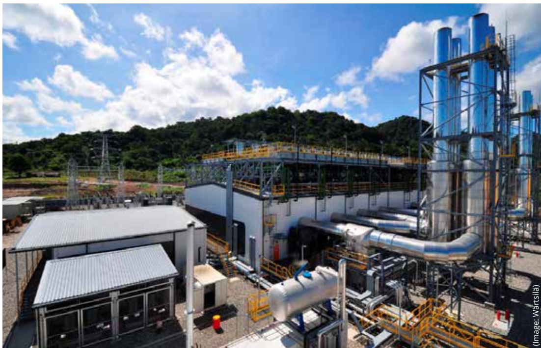
LPG-powered electricity generation
